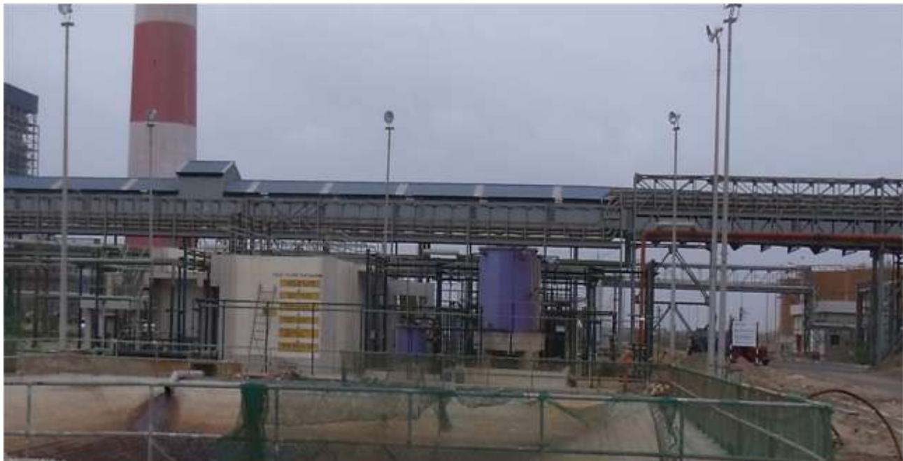
Effluent Treatment Plant (ETP) and sewage Treatment Plant (STP) for treatment of different effluent from Coal pile run off, plant drains and Sewage resp.
