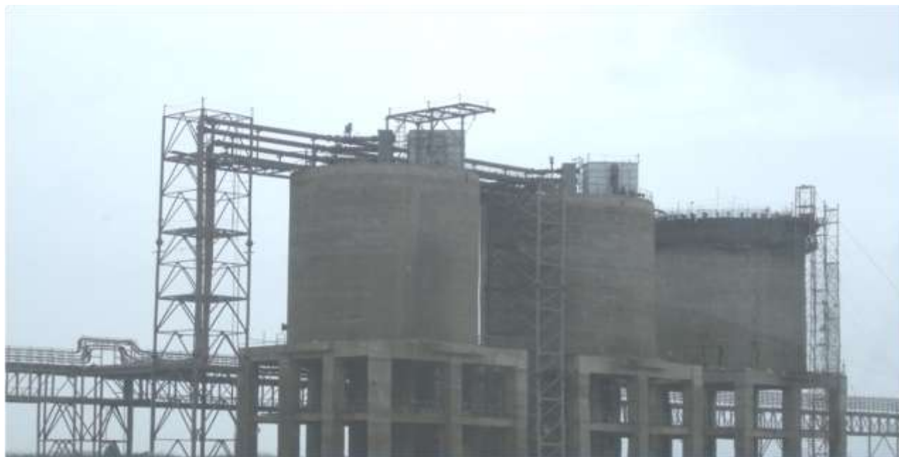
Fly Ash Silo for safe storage of Fly ash and pneumatic conveying system to avoid any fugitive emission during transportation of Fly Ash
