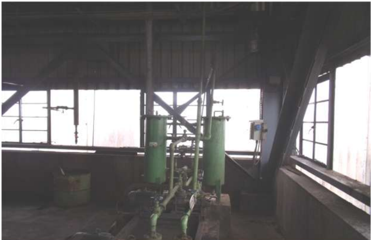
State of the art dry fog system to control fugitive dust from transfer points
